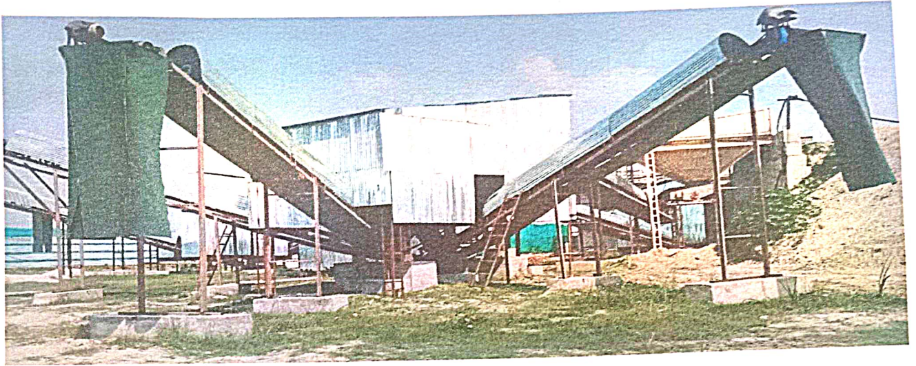
Fig 3 cover the all conveyors
